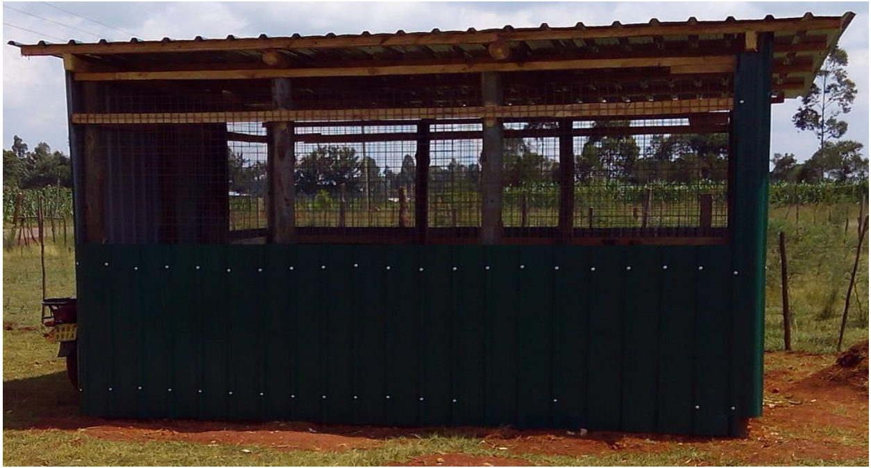
The main kitchen area. Presently putting in the flooring and sink and cutting area. Soon will install four energy saving stoves
