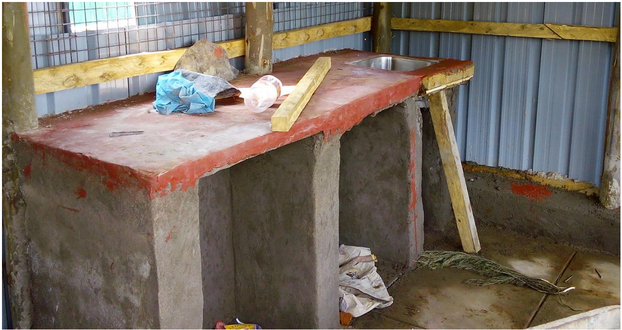
Kitchen cutting and sink area. Note 2 ft. x 2ft. slabs as flooring
